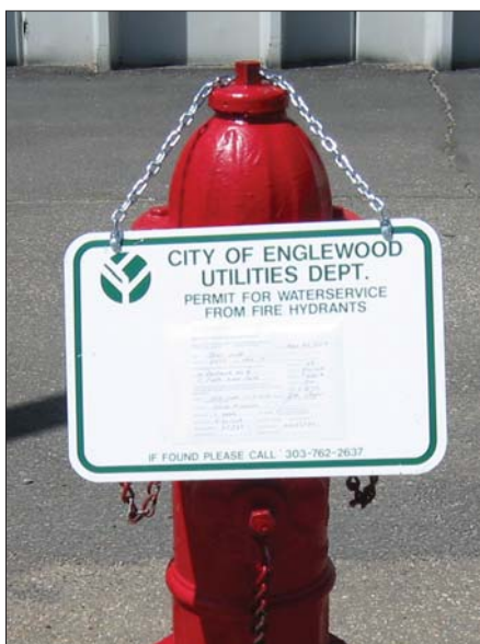
Contractors who use water from Englewood's fire hydrants are required to display a permit approved by the City of Englewood.
